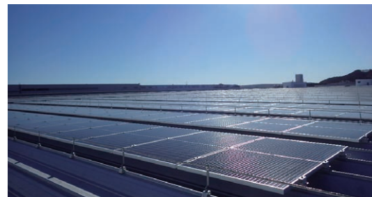
Saitama Factory's Yorii assembly plant (2.0 MW)
