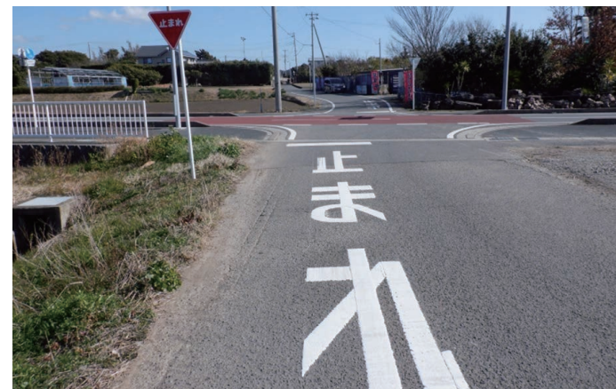
After improvement: The "STOP" line and letters were repainted and colored pavement within the intersection were added.
