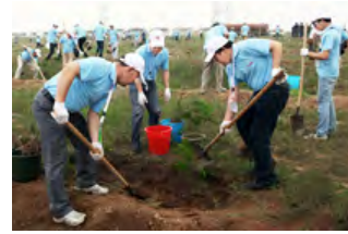
Associates dig dirt to build an embankment and carefully plant seedlings one at a time.
