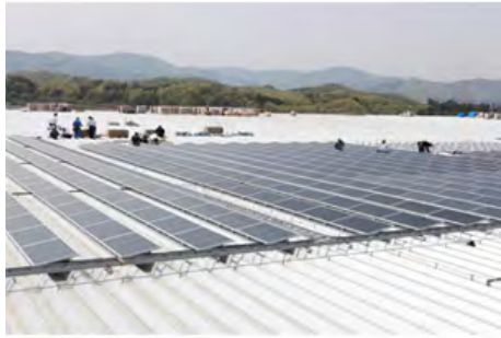
The building's megasolar power generation facility (top)
