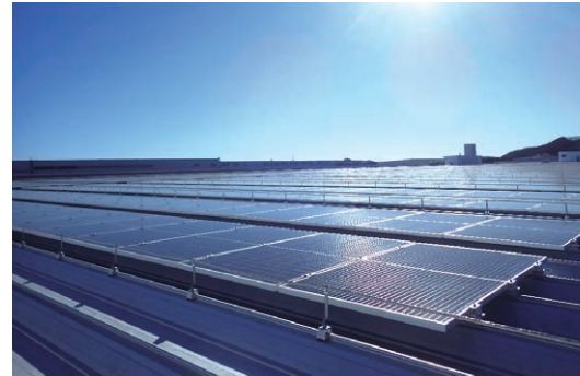
Saitama Factory's assembly plant (2.0 MW)
